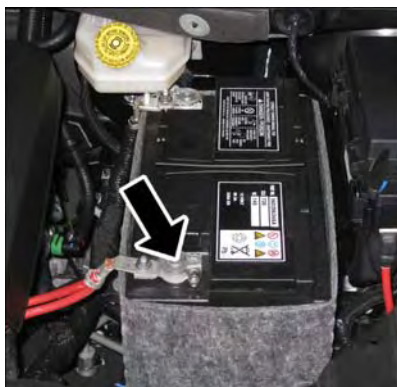
Positive Battery Post
